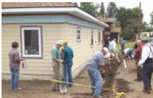
Grace Lutheran Church, with Bishop Tom Aiken, prepare for sidewalk in Ely
